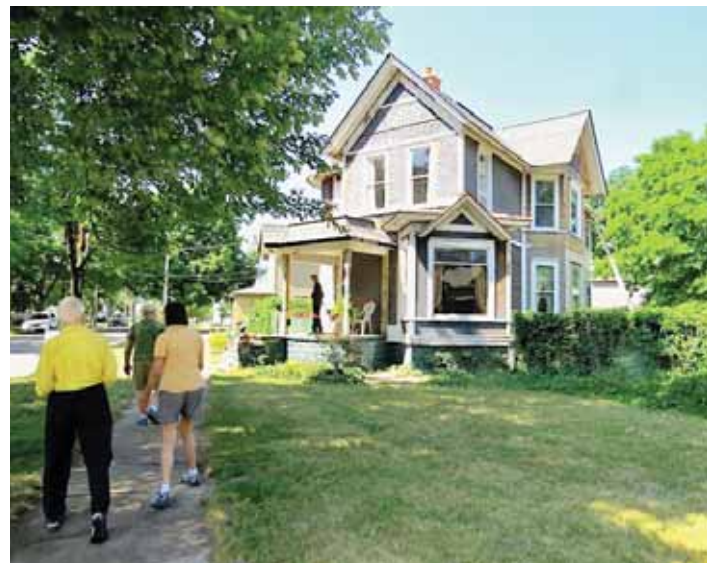
Heading in for a closer look at the restoration in progress at 209 Oak St.
