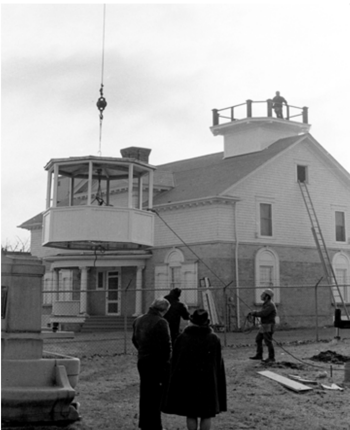
This archival photo taken Feb. 6, 1973, shows the installation of the replica lantern room. Photo provided by Josh McIntyre
