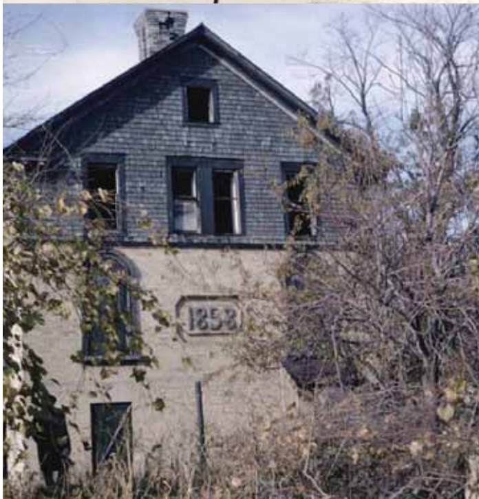
These photos reveal the vandalism and disrepair that befell the building that would become Old Lighthouse Museum. Photos provided by Josh McIntyre.
