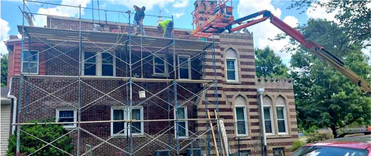
Phase 1 of the Citizens Concerned for the Homeless project involved exterior improvements.
