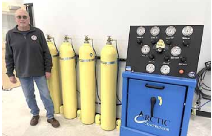
John Wall stands by space designated for the fire department’s self-contained breathing apparatus.
