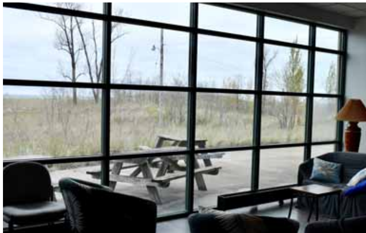
Michigan City Senior Center’s new larger north-facing windows that showcase the beautiful view of Lake Michigan. Photo by Kim Nowatzke.
